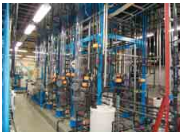
An experimental water treatment plant is used to carry out researches on contaminant removal technologies
