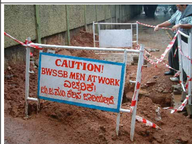
Installation work of DM (district meter) Bulk meters, called district meter, are installed at inlet points of DMAs to measure supply volume to eachDMA.
