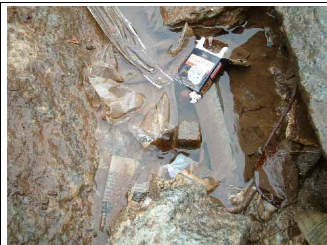
Leakage UFW rate is estimated at 50% of water supply volume
