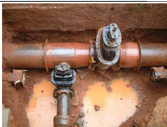
Restructuring distribution networks Based on the hydraulic analysis, restructuring work such as re-connection etc, is being done so as to ensure optimal water pressure within DMAs.
