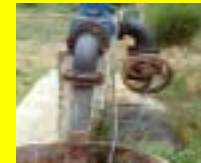
Borehole and pump, managed by village community, Pemba, Zanzibar
