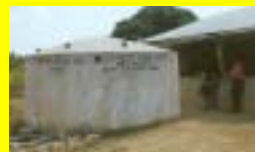
Roofwater harvesting tank, Zanzibar - installed by a donor agency
