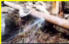
Unreported pipe bursts in Upolu, Samoa
