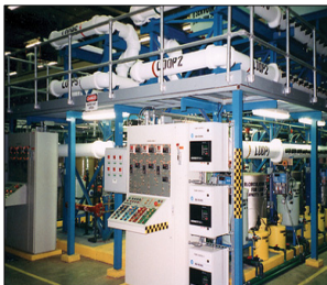
Simulated drinking water distribution system
