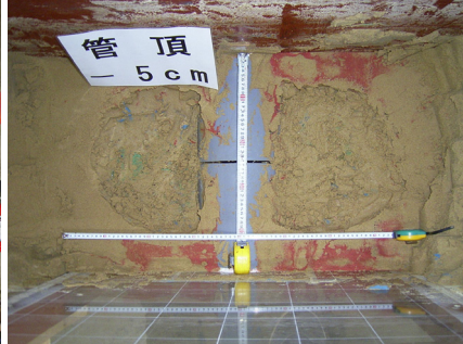
Loosened soil on both sides of crack
