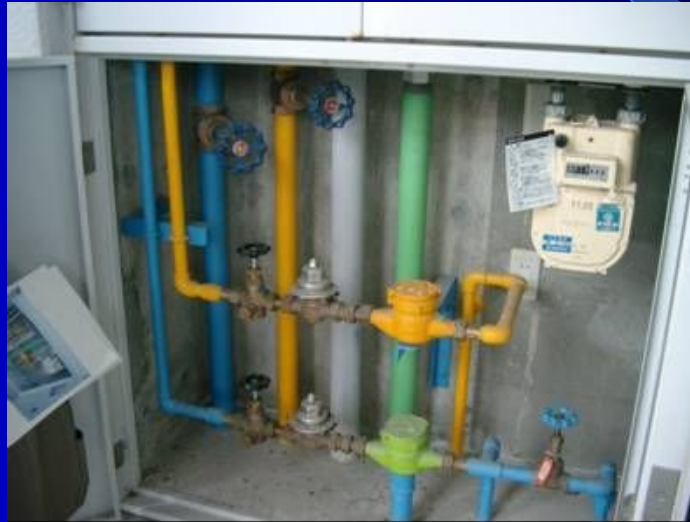
Example of distinction by color-coding the pipes (Yellow is reclaimed wastewater, blue is drinking water)
