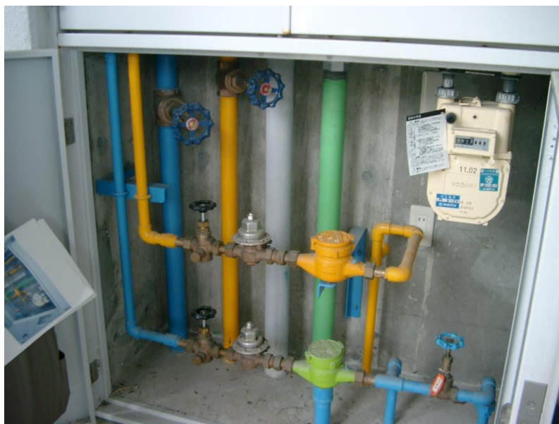
Photo 1 Example of distinction by color-coding the pipes (Yellow is reclaimed wastewater, blue is drinking water)
