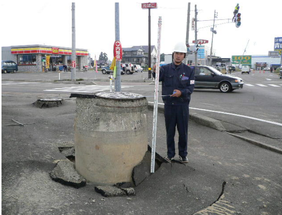
Photo1. A lift-uped manhole in Niigata-ken Chuetsu Earthquake
