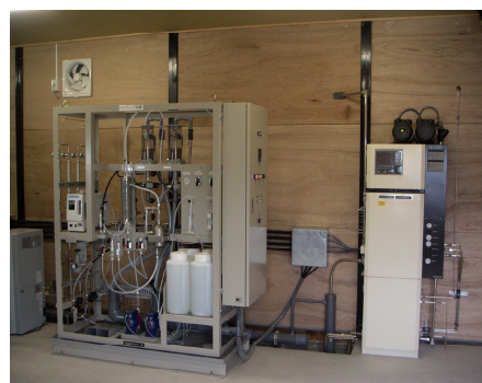
Photo-2 Odor-Causing Compound Detection Equipment (VOC Monitoring System)
